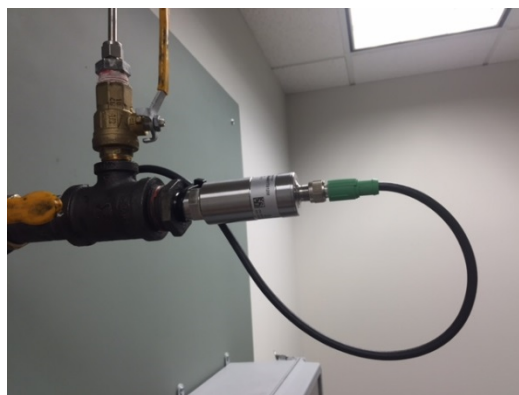
Figure 16 E+E Probe Installed
