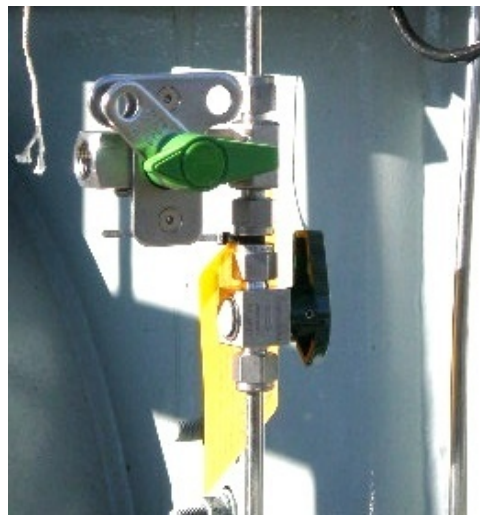
Figure 11: Manual Sample Valve / Secondary Shut-off Valve
