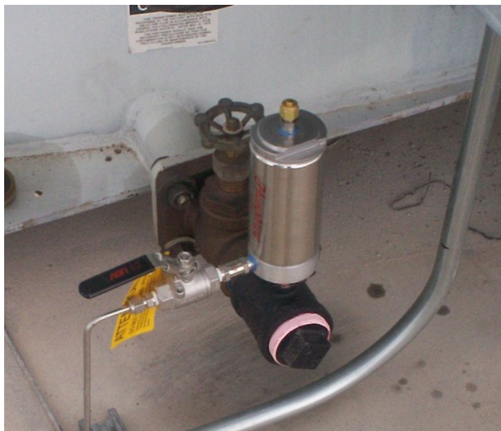
Figure 3: Installed Bleed Fixture
